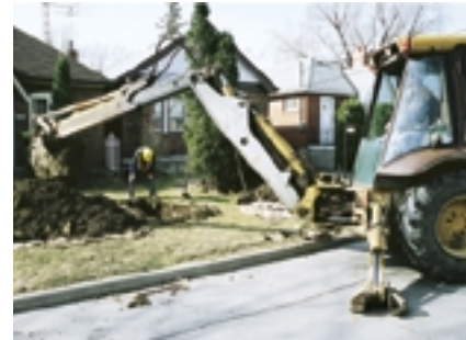
Figure 4.44C This backhoe is digging up a lawn to install a gas pipe. (To see a diagram showing how a backhoe works, turn to page 327.)
